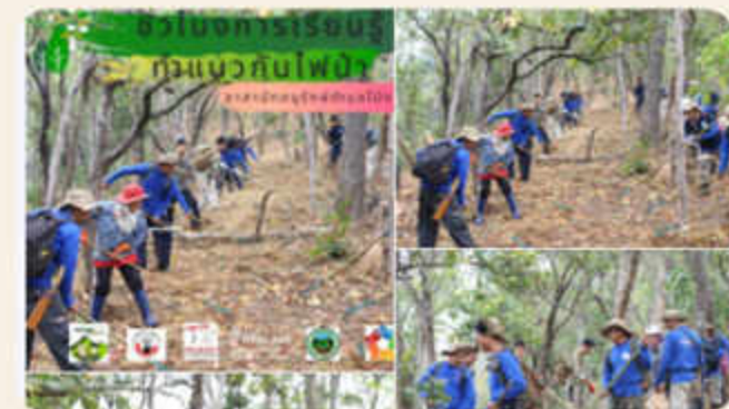
The construction of fire breaks system in order to prevent wildfire of the Volunteers of All Ages Against Wildfire Group at Pong Nam Ron sub-district, Fang district, Chiang Mai province, in cooperation with local communities, Buddhist monasteries, local authorities, and associates from local civil society and private sectors. This project has also supported and encouraged local communities to create their public media space, using their stories, through social media, for example, the Pong Nam Ron Volunteer group of Fang district, Chiang Mai province, presenting the project result and fund raising through their Facebook home page at อาสาป้องกันดับไฟป่า ป่าป๋นน้ำร้อน - ฟาง PNR Fire VolunteerS | Facebook .
